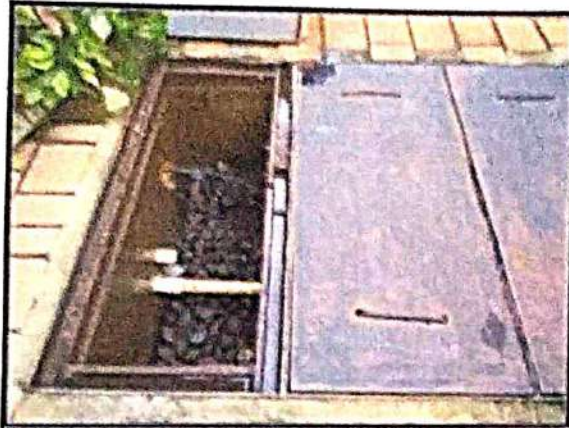
Rainwater Harvesting System- Recharge Pit
