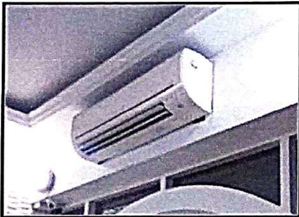
Air Conditioners Installed in Lab
